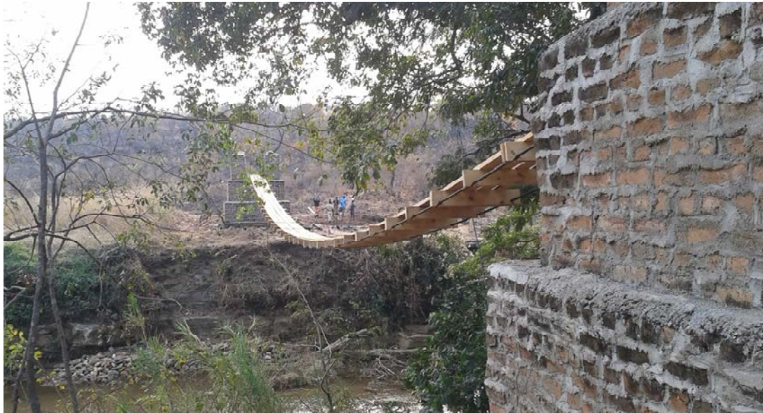
Figure 19: Uledi bridge as we left it, with decking replaced but no handrails
