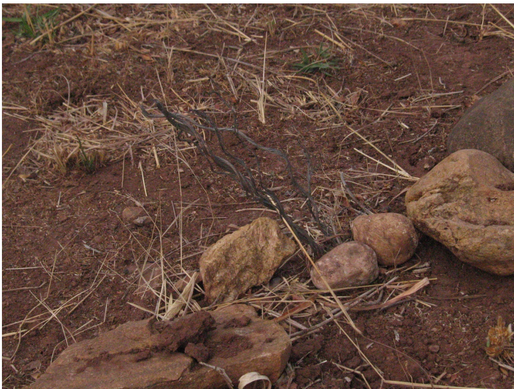
Handrail cable cut through just above embankment level
