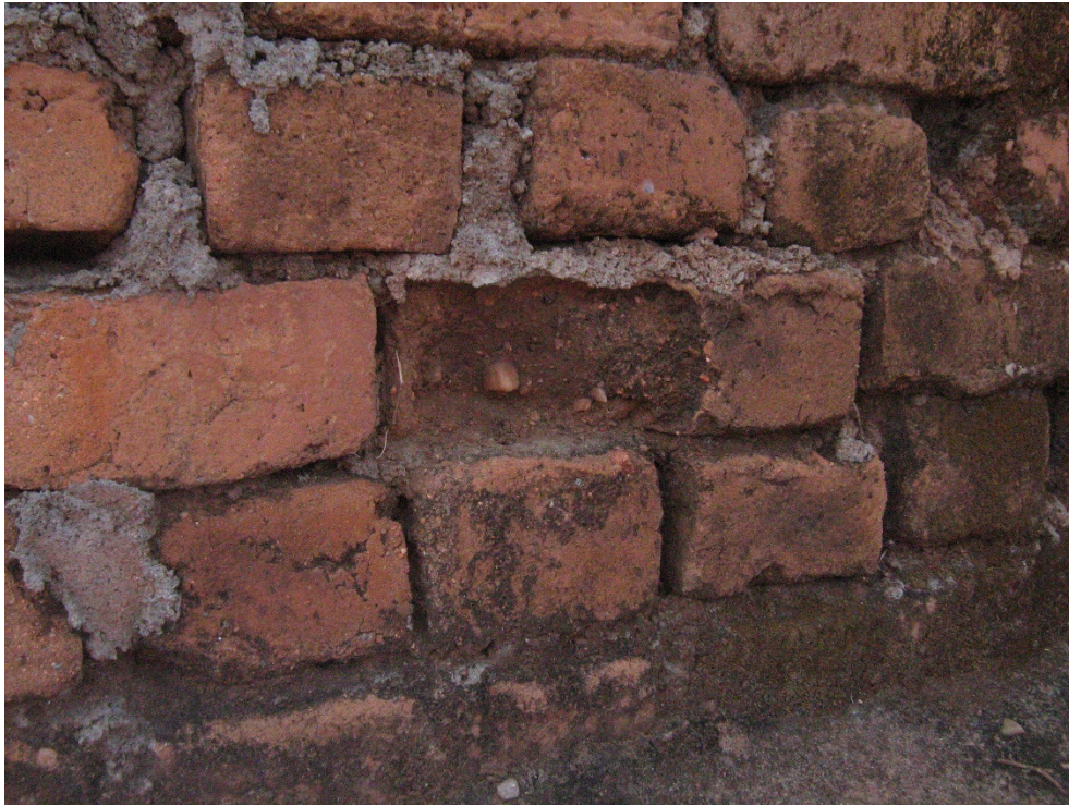
Brickwork on left tower, in need of repointing
