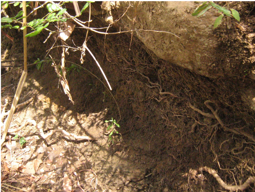
Erosion below left tower
