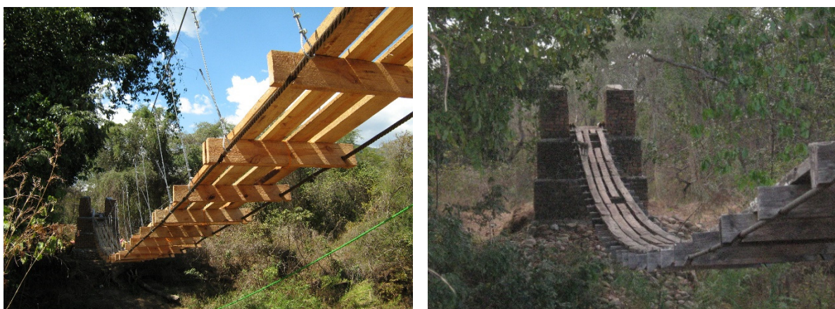
Figure 10: The bridge as we left it in 2007, and as we found it in 2015
