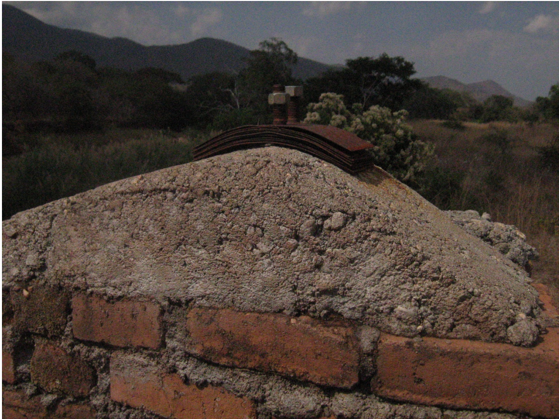
Saddles in good condition
