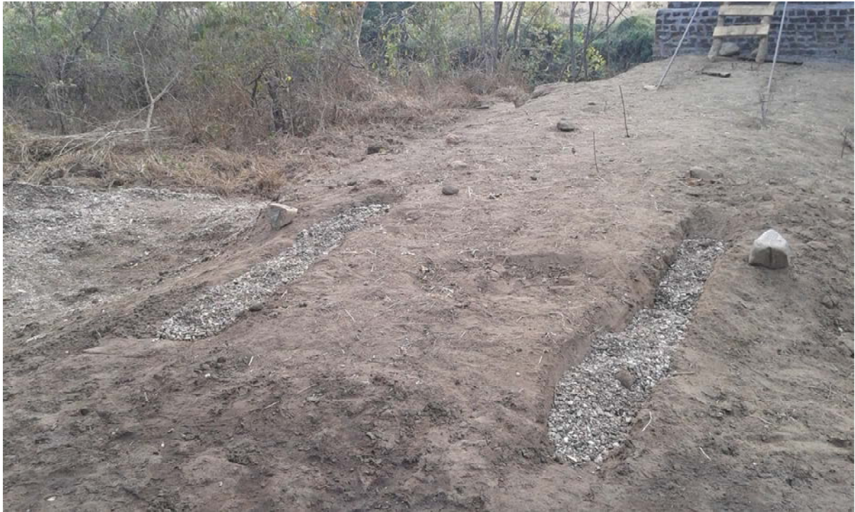
Tranches which will carry new chain handrails have been left infilled with gravel as a temporary measure.
