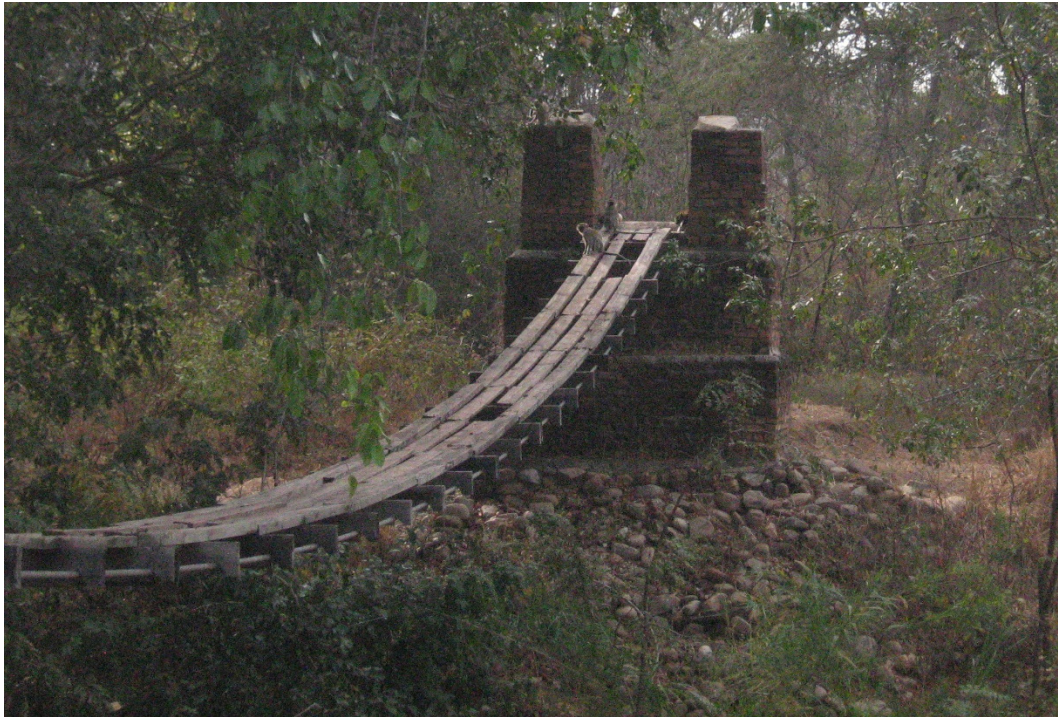
View of bridge from left bank – showing missing handrail cables and rotten decking
