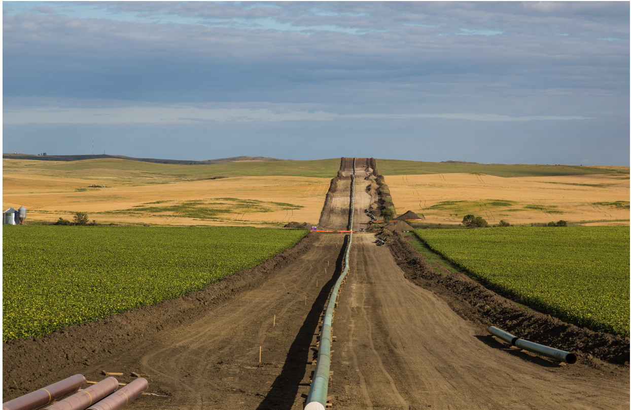
Bakken Dakota Access Oil Pipeline, August 25, 2016. Photograph by Tony Webster https://creativecommons.org/licenses/by-sa/2.0/ https://www.flickr.com/photos/diversej/29357938502
