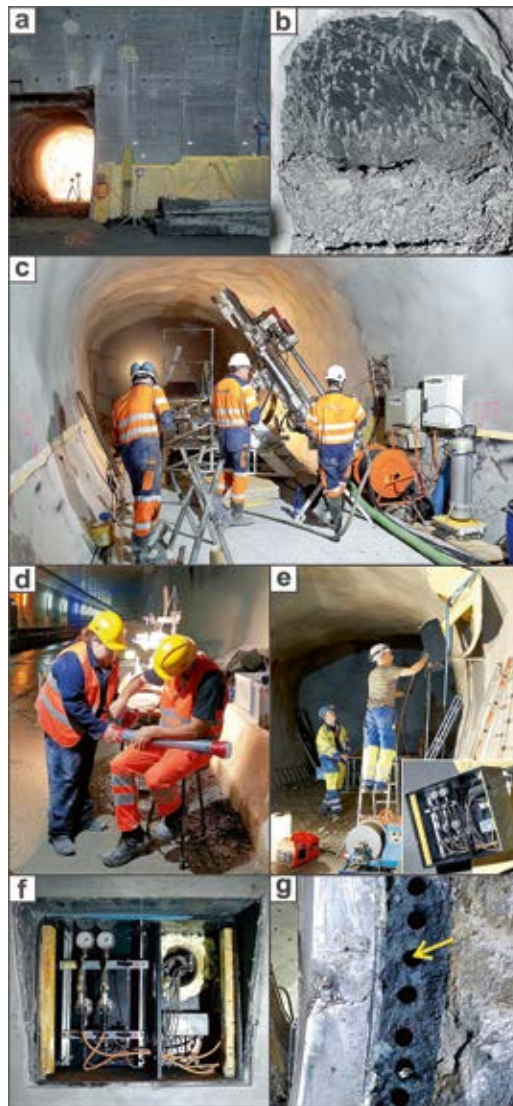
Figure 2: Photographs showing (a) the cross-passage 5a located between 6.3–11.3 m north of the measuring section (MS; see Figure 3), (b) unsupported face of the cross-passage 5a, (c) directional dry drilling of CP-2 and equipment for hydraulic testing at the right side of the photograph, (d) sealing of lined cores shortly after drilling by M. Williams and C. Soares, (e) installations of a double-packer system for pore pressure measurements in borehole CP-4 and of the data acquisition and hydraulic control system into a box mounted on a standpipe (lower right corner), (f) final situation of the box inside the inner cast-in-place concrete liner, and (g) drilling of short ( <1 \text{ m} ) boreholes for extraction of annular gap grout specimen.
