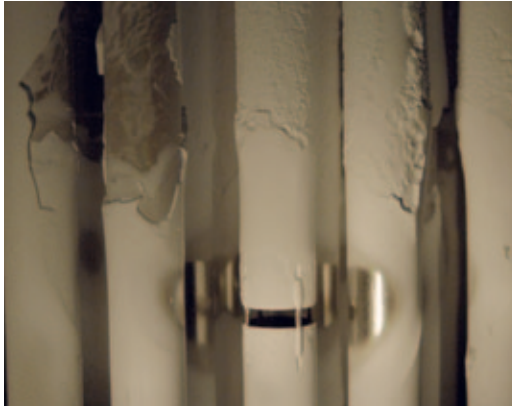
Figure 3: A photograph of the break and the tubes showing thick deposits, and particle-free areas in the closest tubes facing the break.
