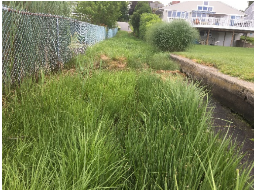
Figure 1: Source 5-013, a seep at the end of a right-of-way at extension of Chace Avenue.
