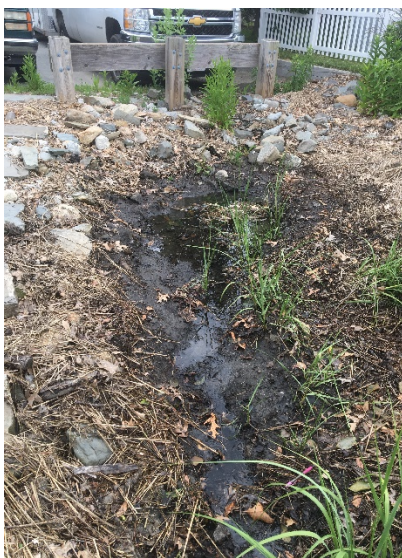
Figure 2: Source 5-030, 18” corrugated metal pipe at the end of Smith Street, Warren, RI.
