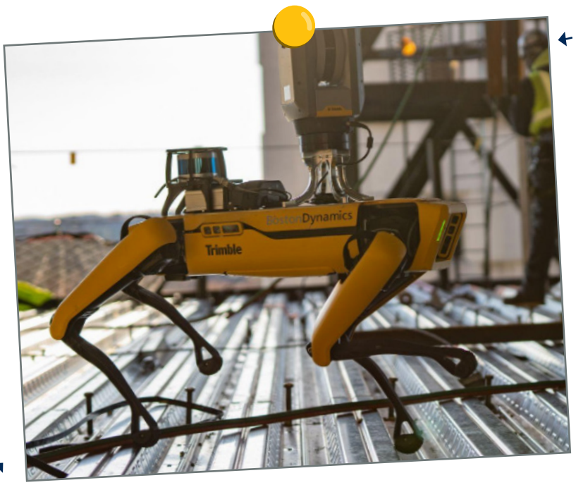
A Spot robot monitors a construction site. (Photo courtesy of Boston Dynamics)
