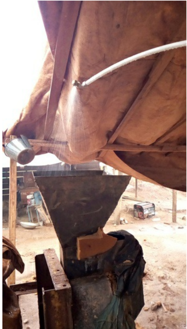
Water spray misting installed at ore processing machine.
