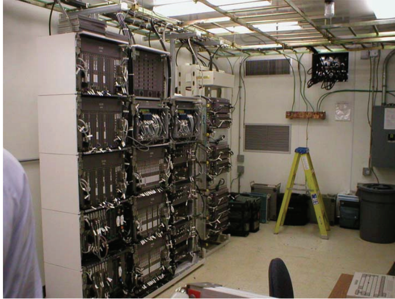
Figure 3-4. Cellular Base Station Equipment
