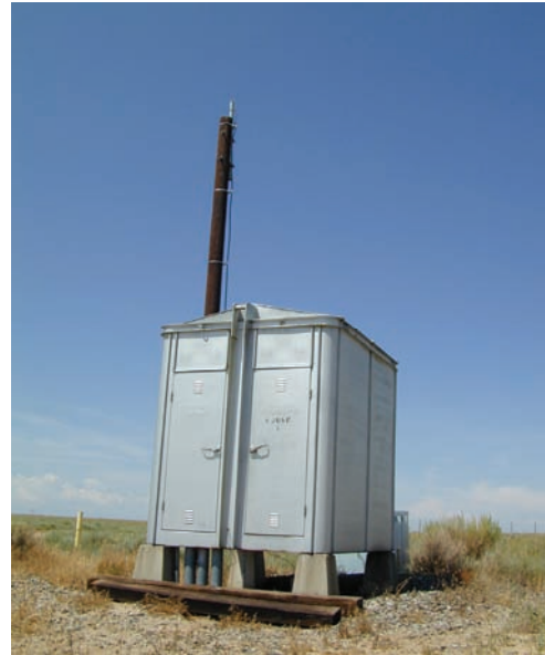
Figure 6-3. Typical Block Signal Control Equipment Enclosure
