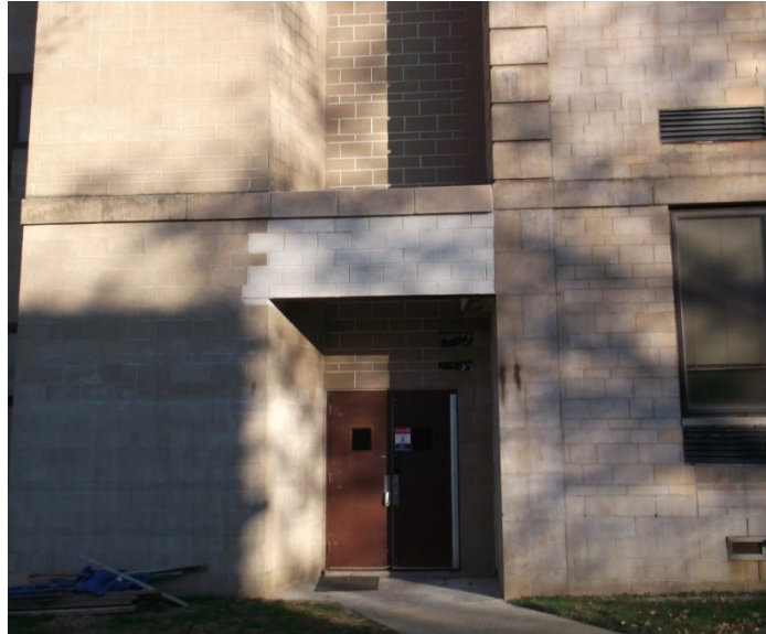
Figure 2. Evidence of Contractor's Use of Incorrect Materials for USMMA Academic Building Renovations
