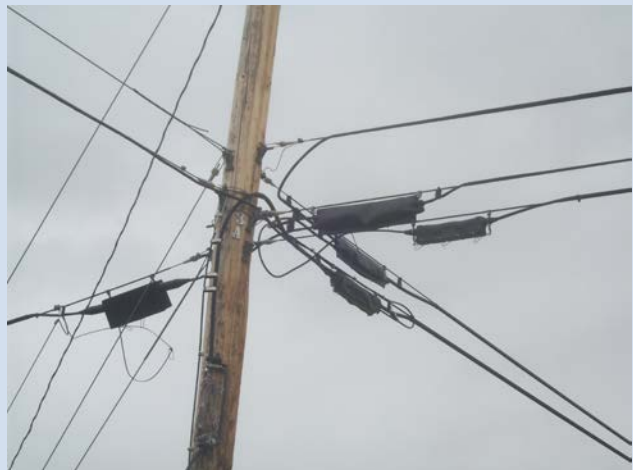
Aerial Coaxial Cabling in Dinosaur
