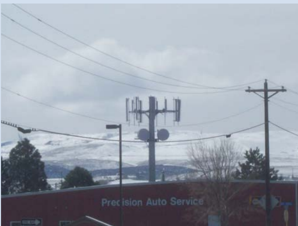
Cellular Antennae with Microwave Backhaul
