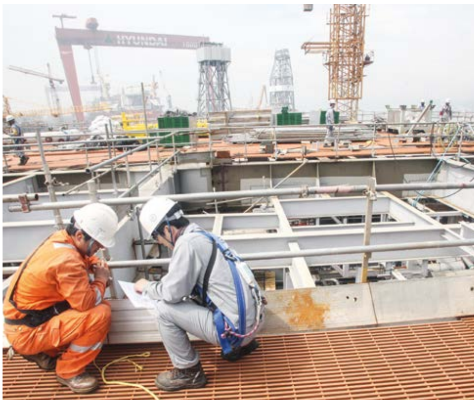
Contractors construct a platform in South Korea for our Clair Ridge project in the UK North Sea.
