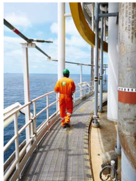
▲ The monitoring stations around our vessels in Angola are designed to be in place for 25 years.
