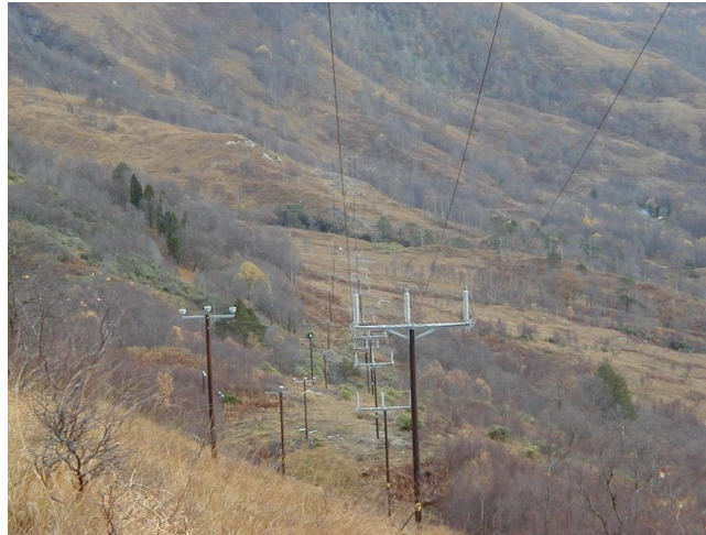
Figure 23: 33 kV and 132 kV Overhead Lines on the Scottish Mainland (Photograph courtesy of SSE)
