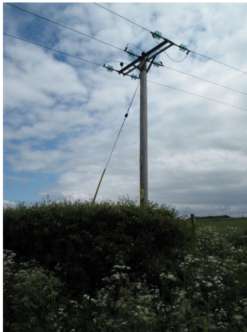
Figure 13: 11 kV Line in Caithness
