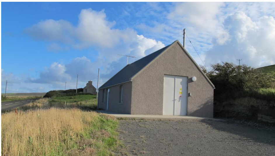
Figure 9: Hammars Hill 33 kV Substation on Orkney West Mainland Serving the Hammars Hill 4.5 MW Onshore Wind Farm (Cables Run Underground from the Turbines to the Substation Building)
