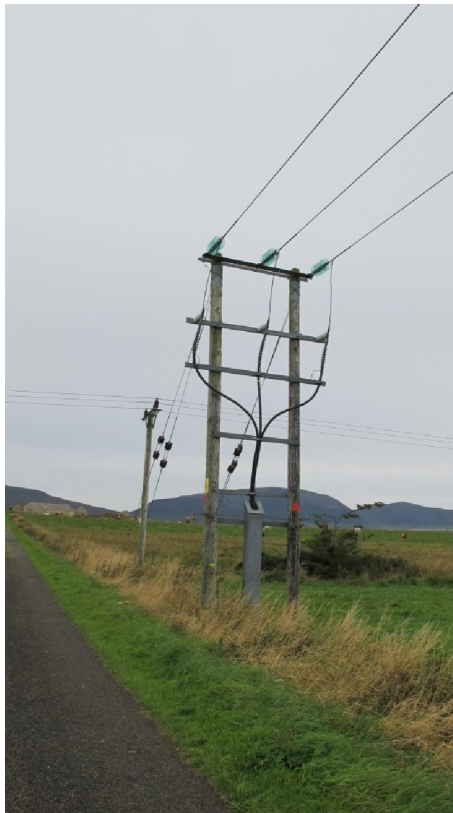
Figure 7: 33 kV Line on Orkney at the Point at Which it Transfers from Underground Cable to Overhead Line
