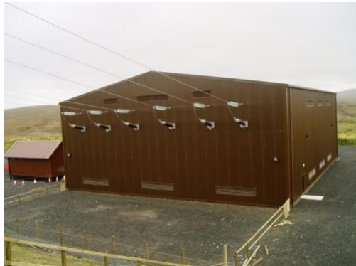
Figure 18: Example of a 132 kV Indoor Substation with Woodpole 'Trident' Overhead Line. (Photograph courtesy of SSE)
