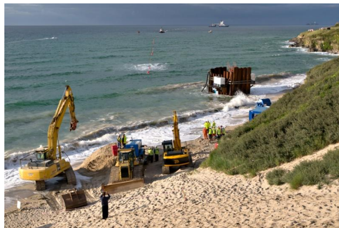
Figure 5: Cable landing works at Wave Hub in Cornwall (high tide) (Photograph courtesy of Wave Hub)
