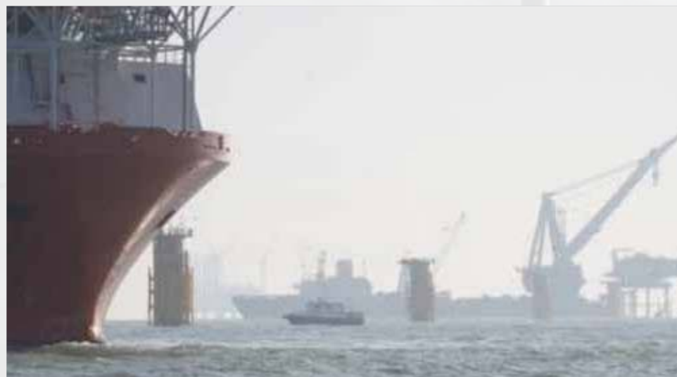
This is the Thanet Offshore Wind Farm being built. Like any construction site, it's a busy place and it is a big challenge to coordinate the many vessels.
