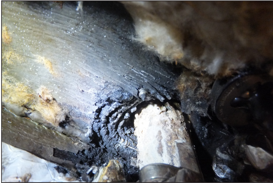
Figure 2: Scorching of the plywood underdeck on a similar vessel
