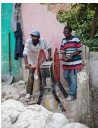
Porky (left) and Elizé (right) crush rubble from the demolished building they are standing in. They are making aggregate that will be used in concrete mix for new buildings.
