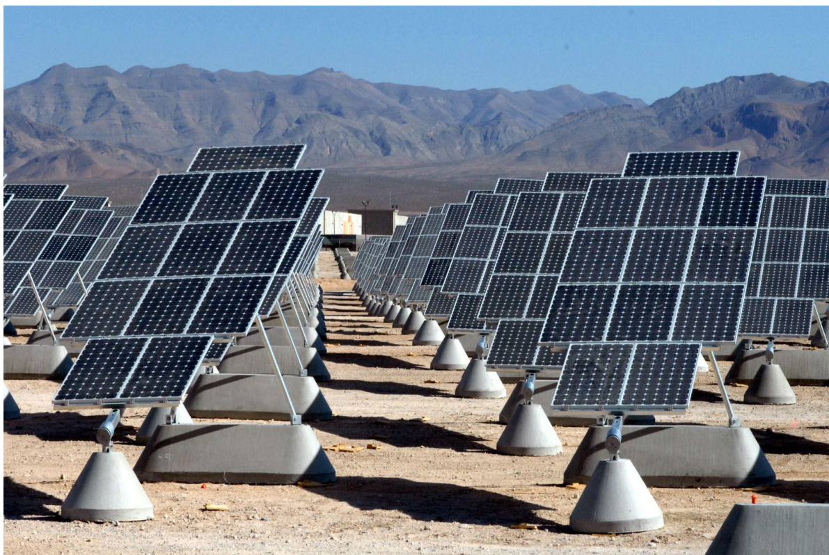
Nellis Solar Power Plant, Nevada. Image source: U.S. Air Force
