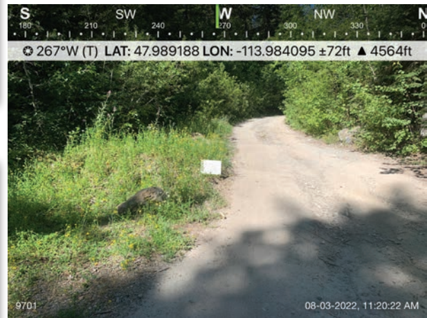
Fig. 15: Flattened earth berm on “closed” road 9701.
