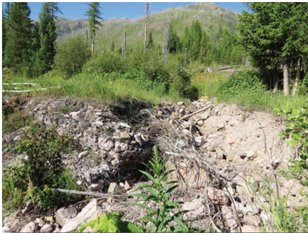
A blown-out culvert in the long-closed Bunker Creek Road 549 in 2014, upstream of bull trout critical habitat.
