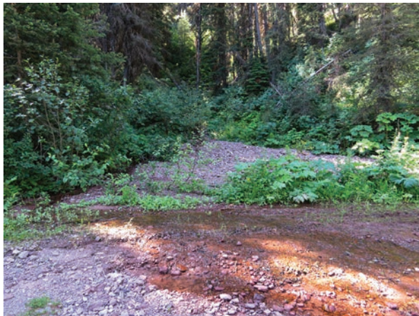
Road 1673 looking upstream at plugged catchment.
