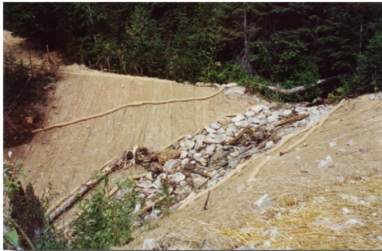
Road decommissioning removes culverts, restores streambed gradients, removes road fill, and stabilizes slopes. Paul Harvey photo
