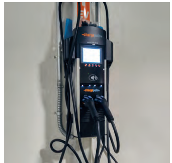
USAID's dual-port EV charging station in the garage of its USAID Annex Headquarters facility in Washington, D.C. PHOTO: USAID
