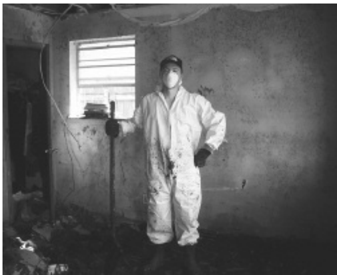
A volunteer helps clear the toxic mud from a home in Chalmette. Courtesy of the Louisiana Bucket Brigade.
