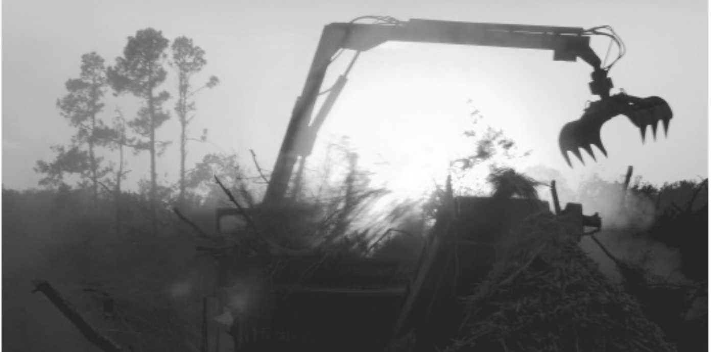
Downed trees are mulched by Ashbritt at a Mississippi dump site. Photo by cottergarage under Creative Commons license.
