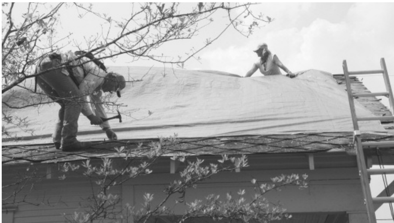
Local church volunteers install a blue tarp for free for a neighbor in Mississippi. Photo courtesy of FEMA.
