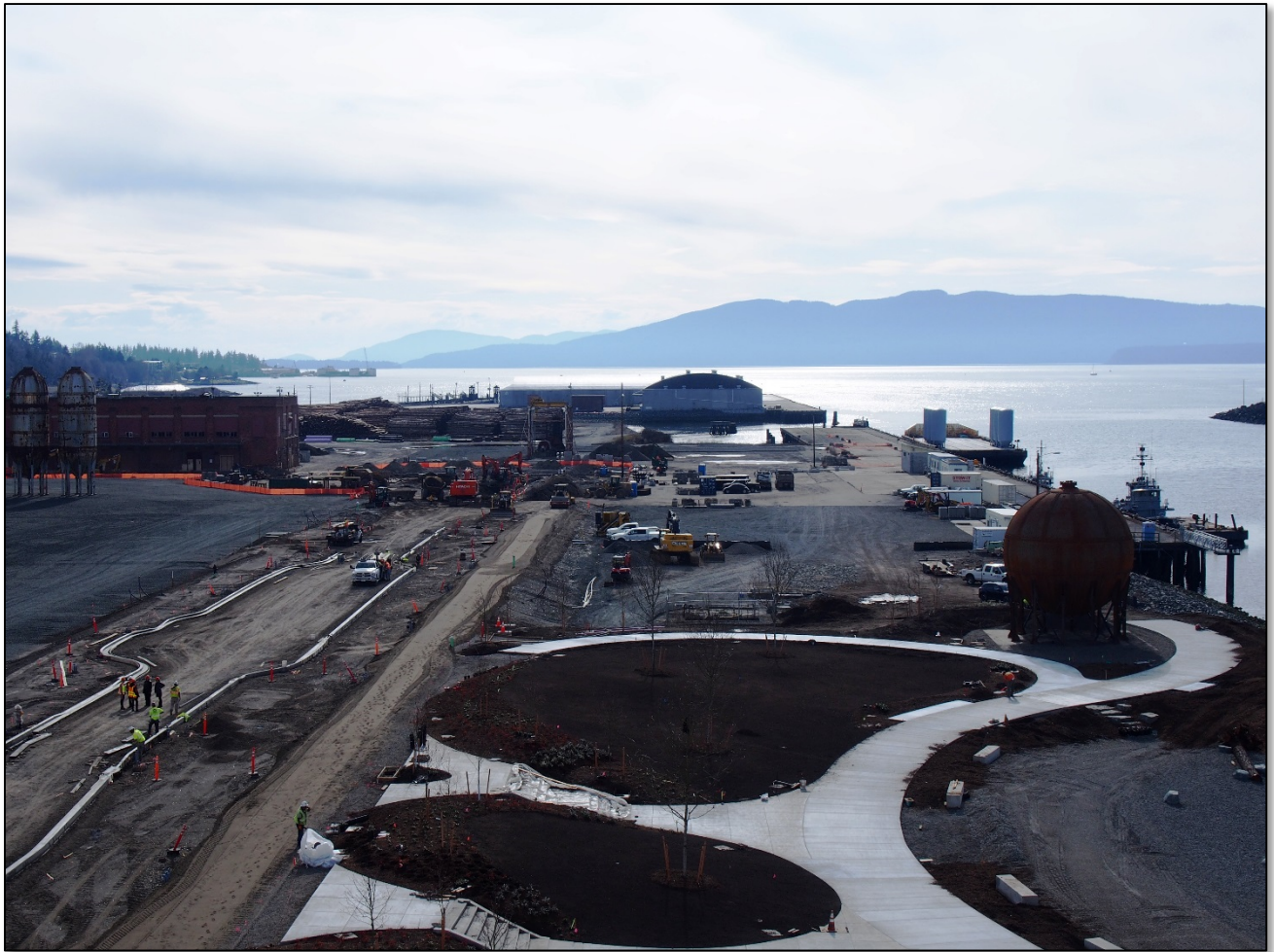
Southerly view of Granary Avenue and Laurel Street under construction, March, 2018. Wide sidewalks and a cycle track along Granary Ave. and Laurel Street will connect to the network of recently completed trails in Waypoint Park.
