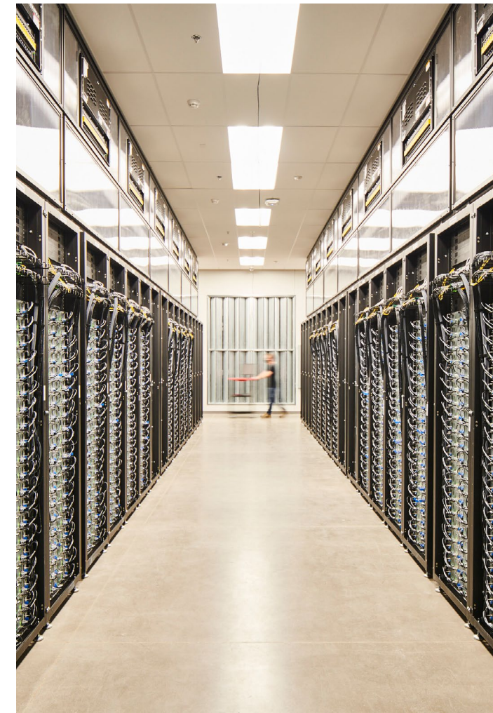
Apple's Reno data center, opened in 2012, takes advantage of the mild climate by cooling its servers with outside air whenever possible.
