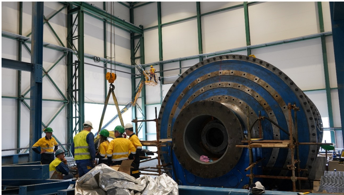
Figure 12: Ball mill, grinding building, July 2023
