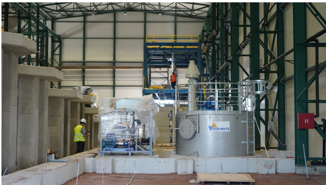
Figure 13: Lime system, flotation building, July 2023
