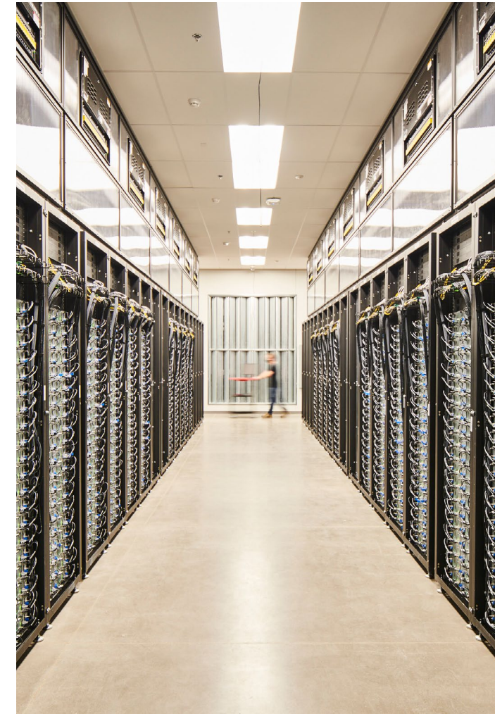
Apple's Reno data center, opened in 2012, takes advantage of the mild climate by cooling its servers with outside air whenever possible.
