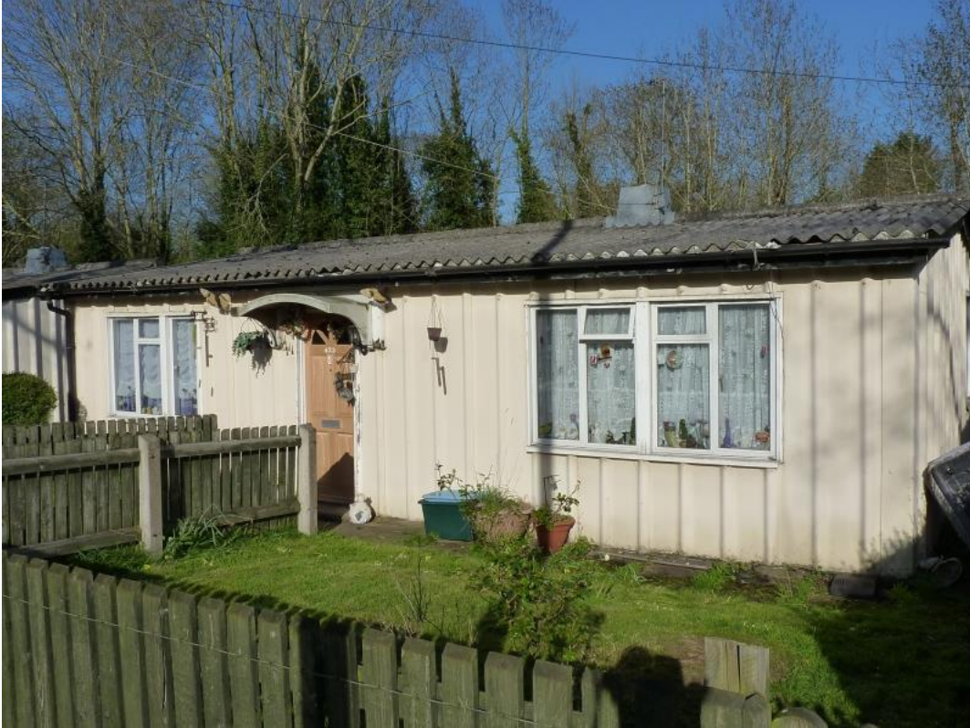
Grade II listed Phoenix prefab at 423 Wake Green Road. Source: Richard law via https://www.geograph.org.uk/photo/5794413
