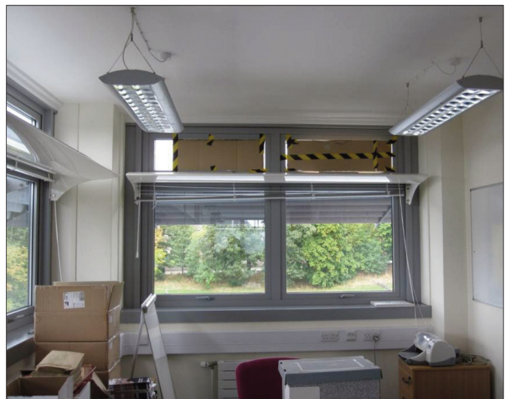
Some building users found it necessary solve glare problems by fitting sheets of cardboard to the toplight.
