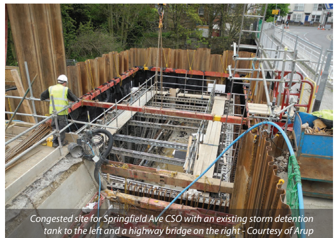
New final settlement tank being constructed within the existing Bridlington WwTW - Courtesy of Peter Smith Photography
