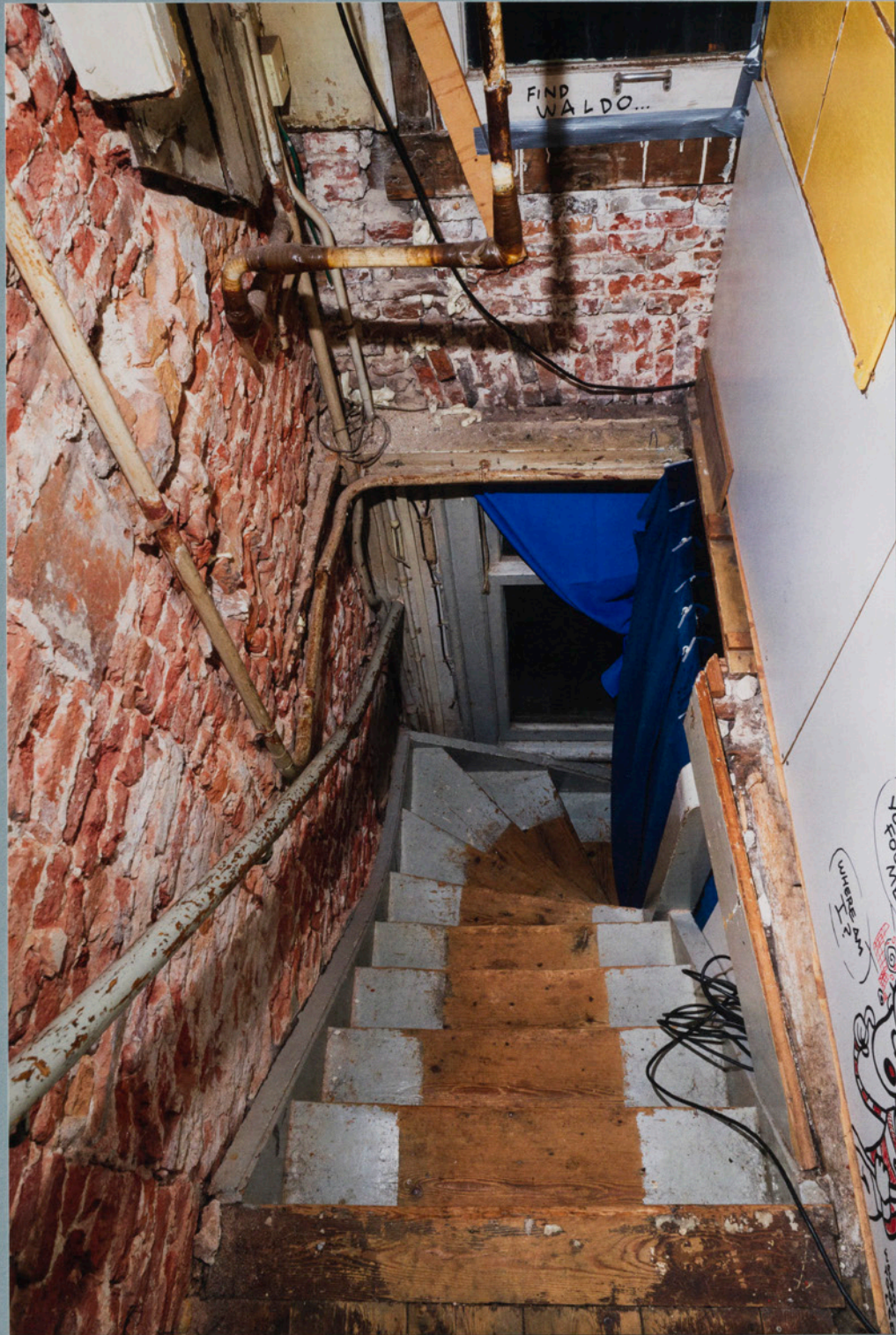
Renovation – As the owner tore down all the internal walls, the squatters had to improvise and rebuild the entire interior by themselves.
