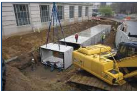
80,000 gallon capacity vault stormwater storage @ National Museum of Natural History
