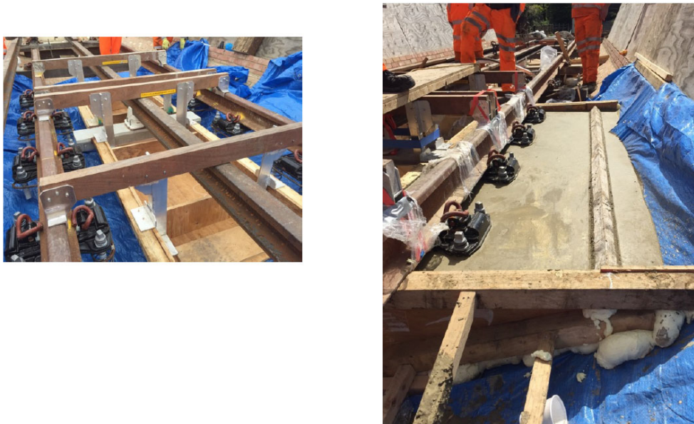
Figure A10.1 –Surface mock-up of the planned rail replacement for Baker Street to Finchley Road underground stations.
