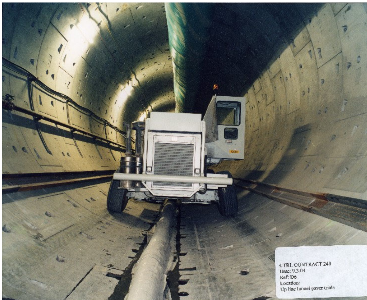
Figure A6.1 Gomaco paver getting ready to provide stage 1 track bed on High Speed 1 in the UK
