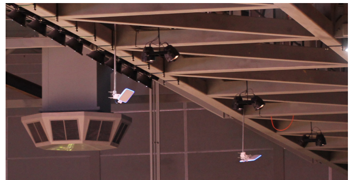
UniFi BaseStation XG hanging below the rafters
