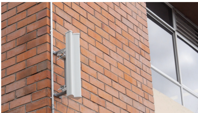
UniFi AP-Outdoor and Sector Antenna for wireless coverage
