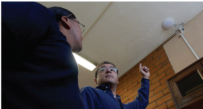
UniFi AP-PRO mounted on the ceiling
