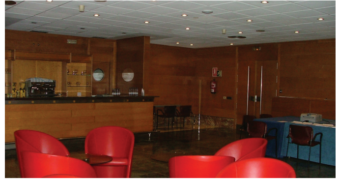
UniFi AP PRO installed in VIP room
