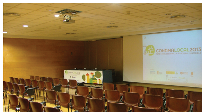
UniFi AP PRO mounted on the ceiling by the projector
