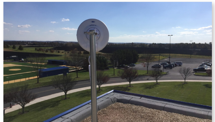
NanoBeam with IsoBeam mounted on building rooftop
