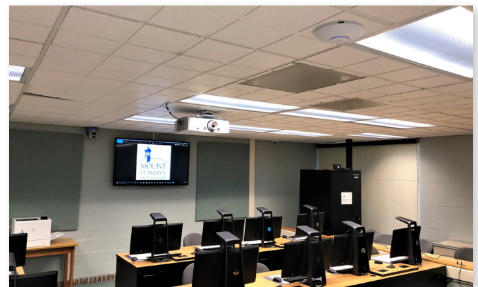
UniFi HD AP installed in computer classroom
