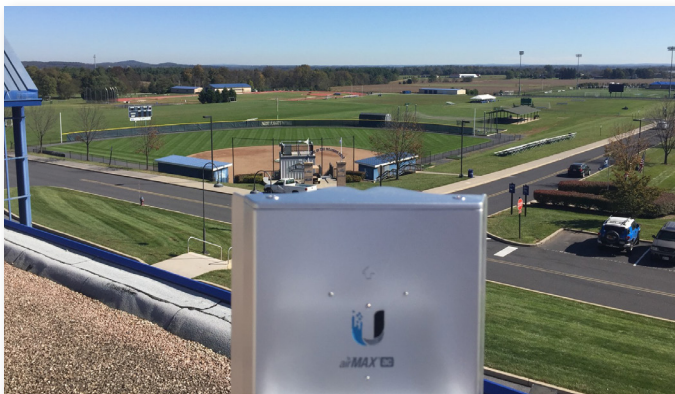
airMAX AC antenna with Rocket5AC Lite overlooking softball field
