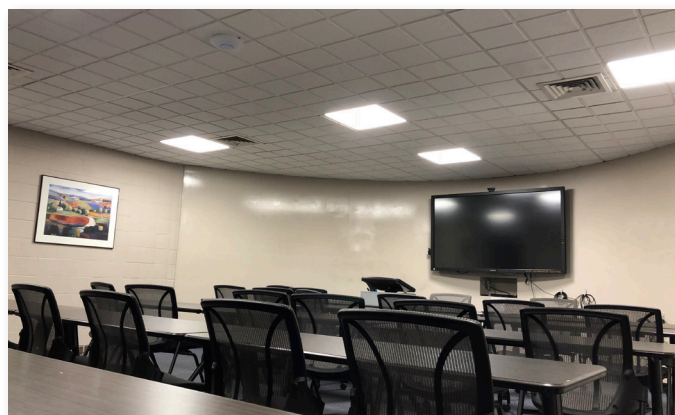
UniFi HD AP ceiling-mounted in classroom
