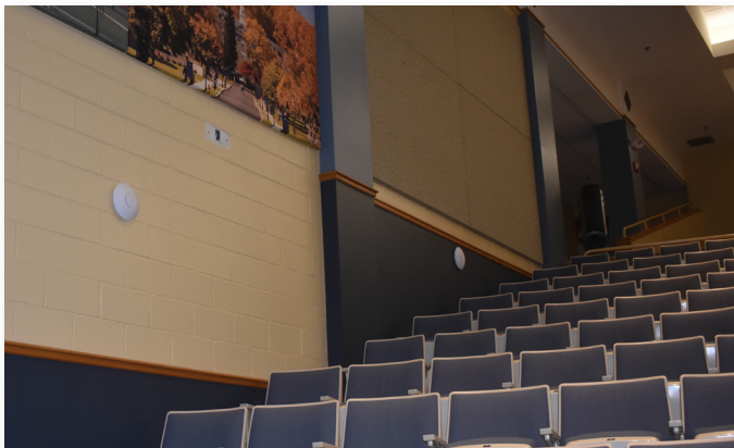
UniFi HD AP installed in lecture hall
