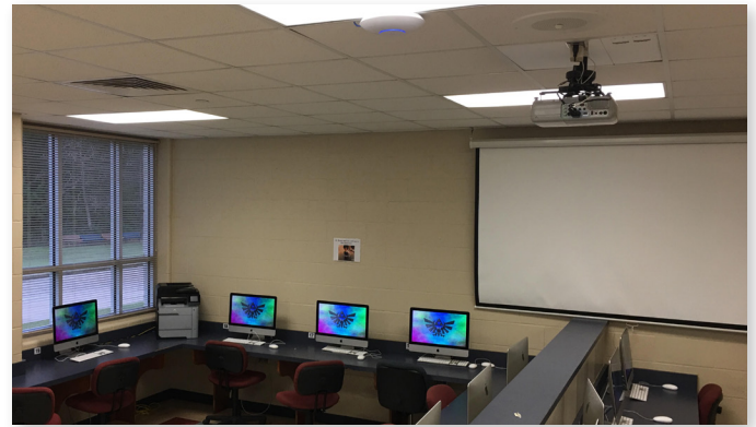
UniFi HD AP installed in high school computer lab
