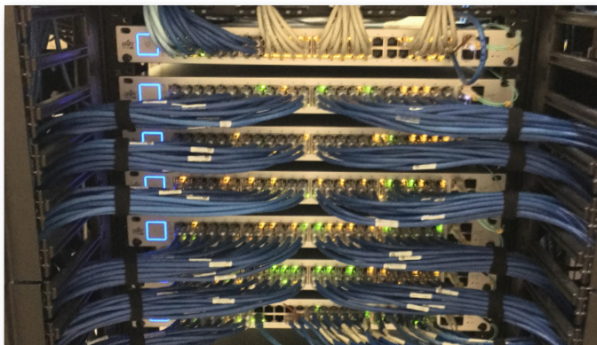
UniFi 48-Port PoE Switches mounted in rack
