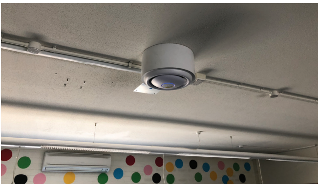
UniFi AC EDU AP installed in a classroom
