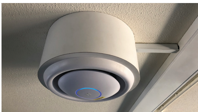
Close-up of the UniFi AC EDU AP in a custom enclosure
