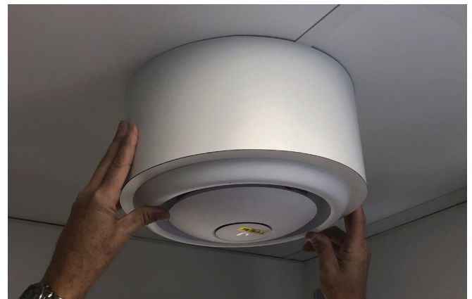
Installing the UniFi AC EDU AP with a custom enclosure
