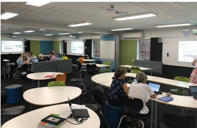
Classroom with UniFi AC EDU AP and UniFi AC Pro AP Installed
