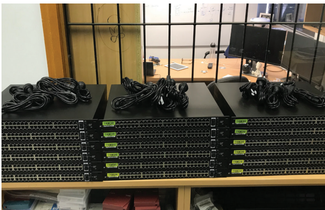
EdgeSwitches about to be powered on
