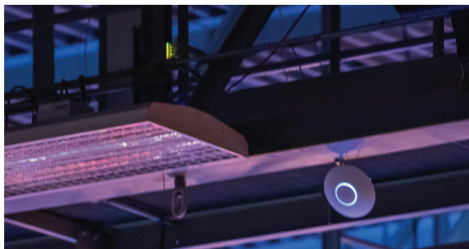
UniFi AC HD AP mounted near arena lighting
