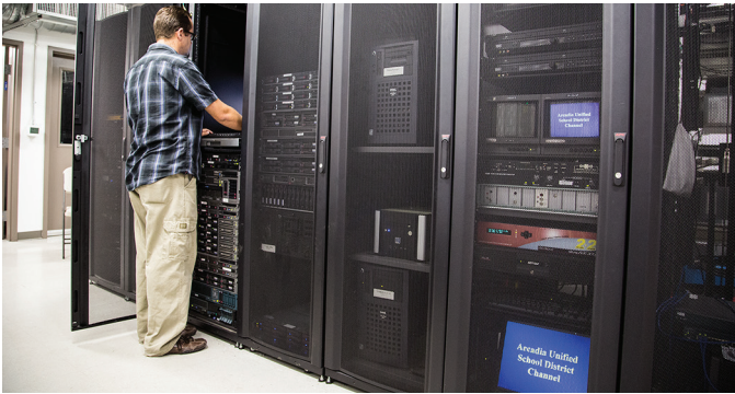
Using UniFi Controller in data center
