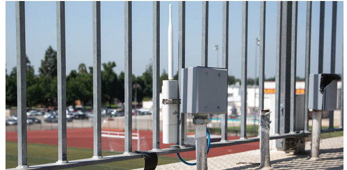
UniFi AP-Outdoor installed outside of stadium press box
