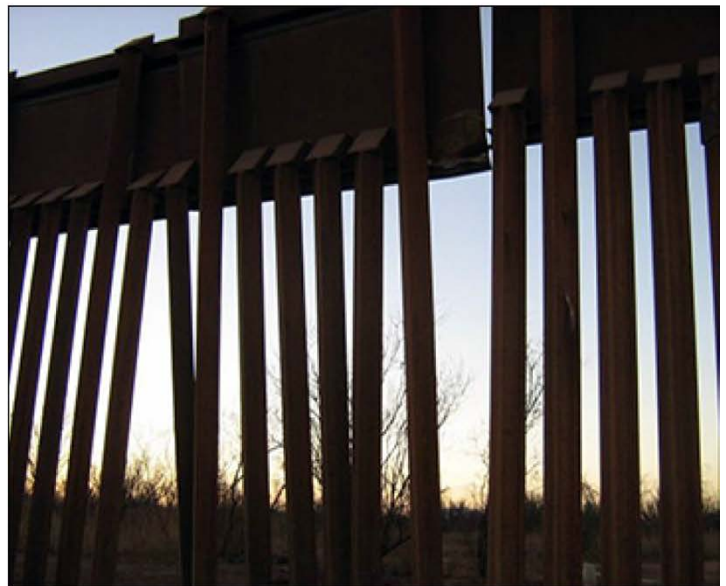
Breach in modern bollard pedestrian fencing
