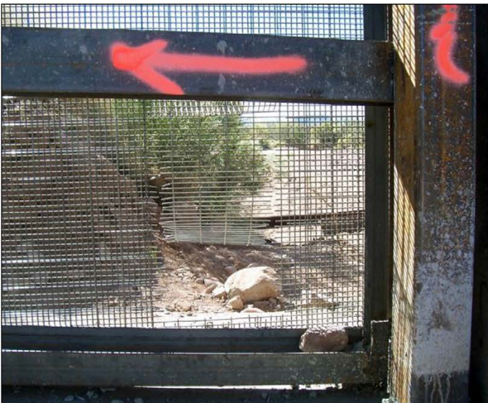
Breach in modern mesh pedestrian fencing
