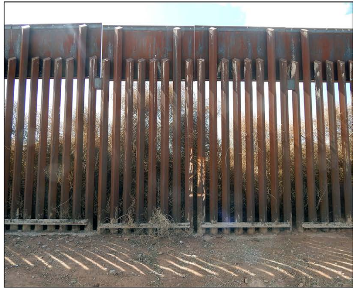
Modern bollard style pedestrian fence
