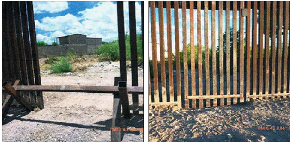
Figure 8: Fence Breach Due To Drive-Through Entry and Subsequent Repair
