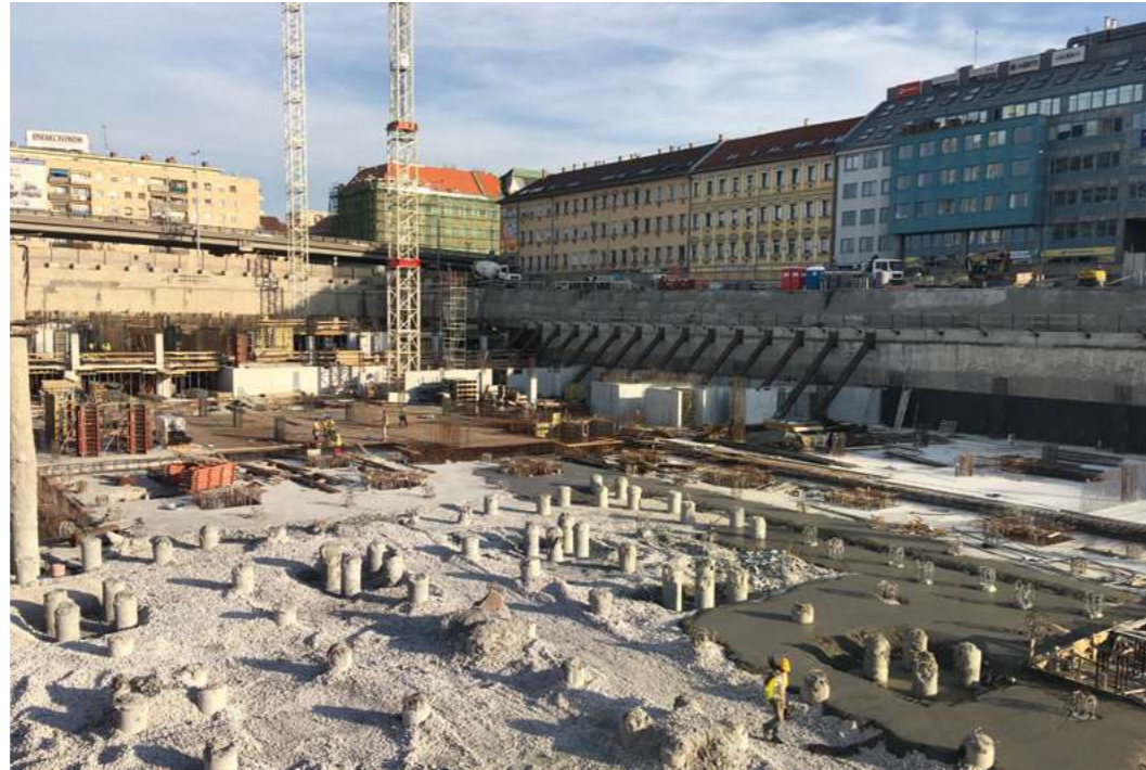
The foundation slab is nearly finished. Agora will soon rise to the street level and above.
