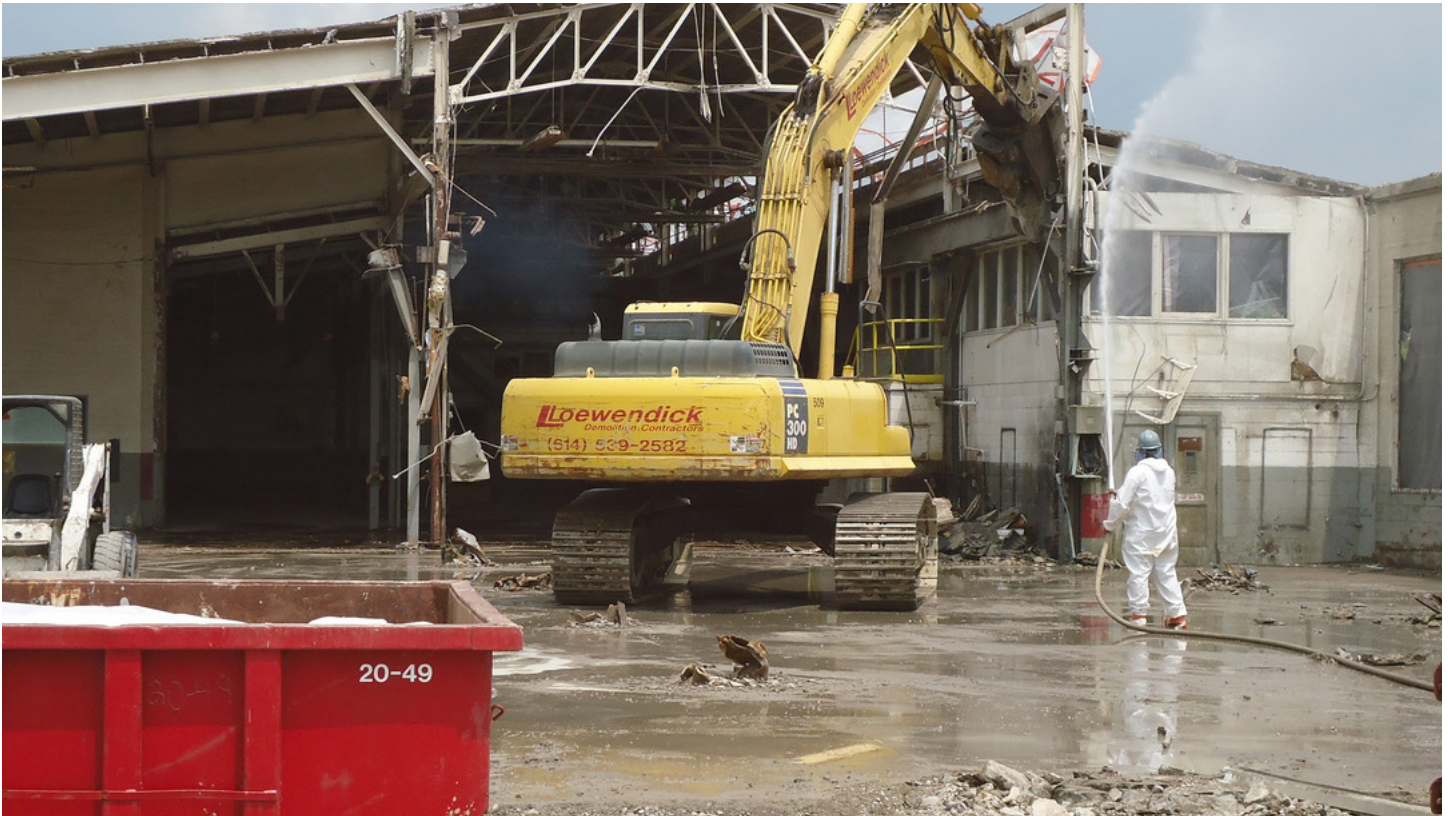
Warehouse Building Demolition for Redevelopment at Wright State University National Center for Medical Readiness in Fairborn, Ohio.
