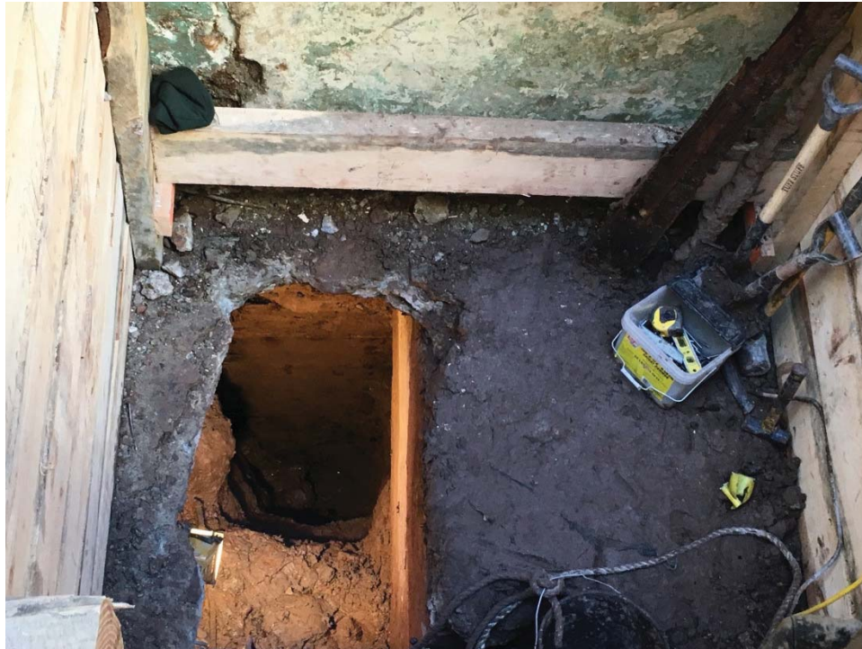
Photo 006: General view of the test pit showing the foundation wall extending to 23 feet below the ground surface, facing south.
