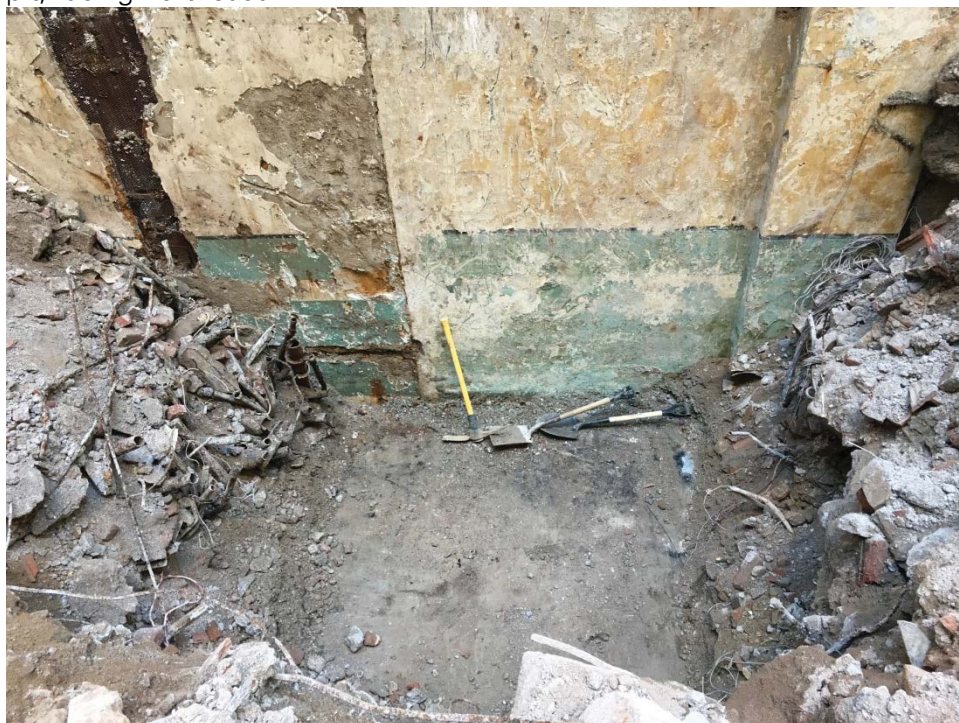
Photo 003: General view of the basement slab encountered at 12 feet below the ground surface, facing south.
