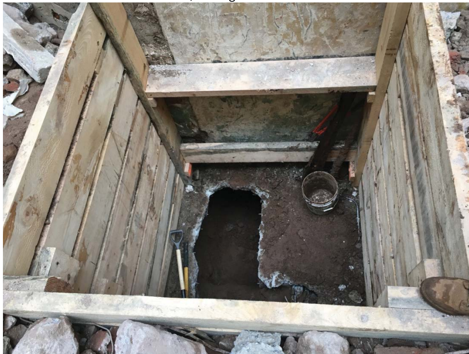
Photo 005: General view of the test pit showing the pile cap encountered, facing south.
