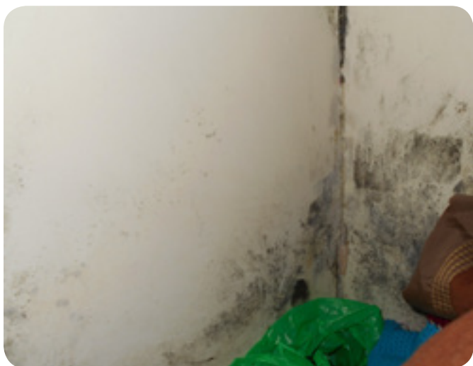
Photograph 1 showing mould behind the bed in Patricia's property.
