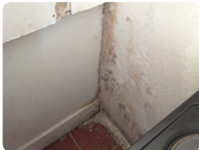
Photograph 3 showing disrepair in Eva's kitchen which made it difficult for her to keep her home clean.
