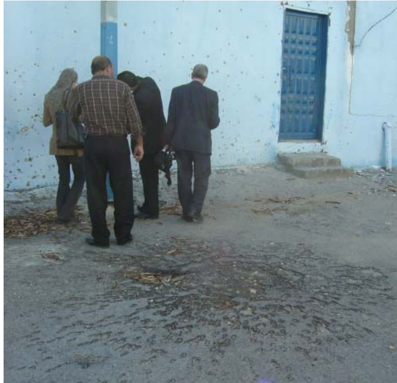
Picture 19: The damage caused from the final shell which hit the headquarters near an exit. The shrapnel damage can be seen on the walls.
