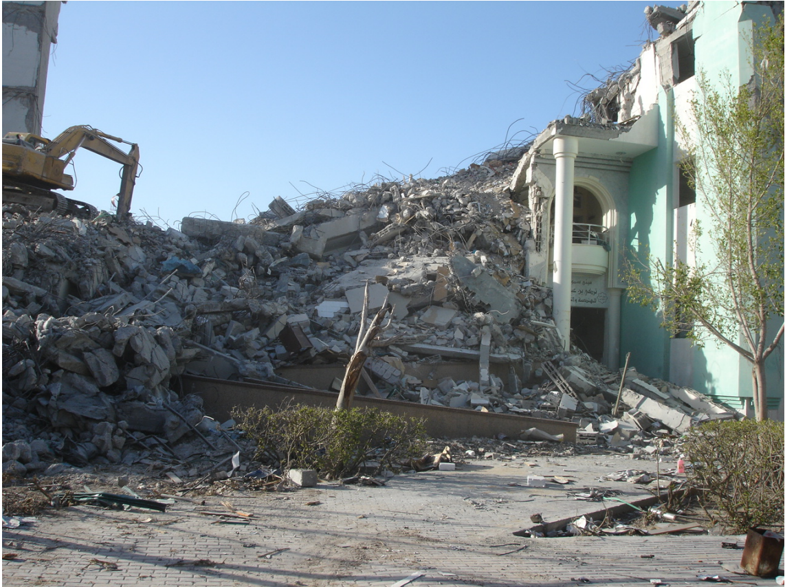
Picture 11: The destroyed Engineering Faculty building.
