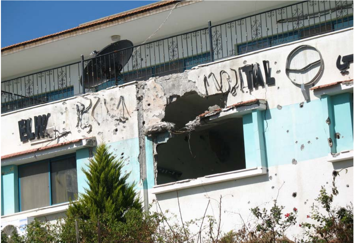
Picture 5: Damage to the Al-Wafa Hospital. The letters “EL W ..... AL” can be seen.
