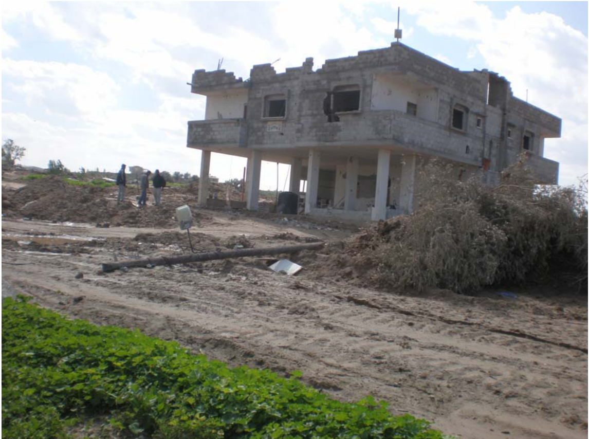
Picture 24: The damage to the Hajjaj family home and the damage to the surrounding land.
