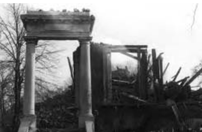
The wreckers. Top and bottom: Sound houses in Brixton Road are demolished for a park, 1978. Centre: A Lambeth Council van acquires an apt graffitto (and two flat tyres) while its occupants destroy a perfectly habitable house round the corner, Radnor Terrace, 1977.
