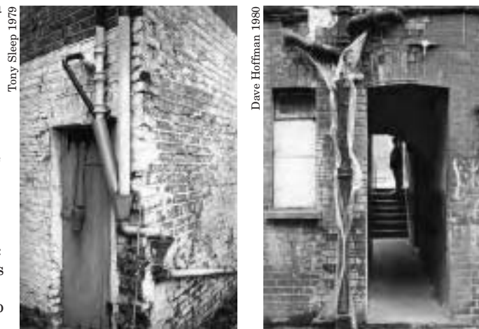
Improvised drainpipes: Freston Road and Fieldgate Mansions
