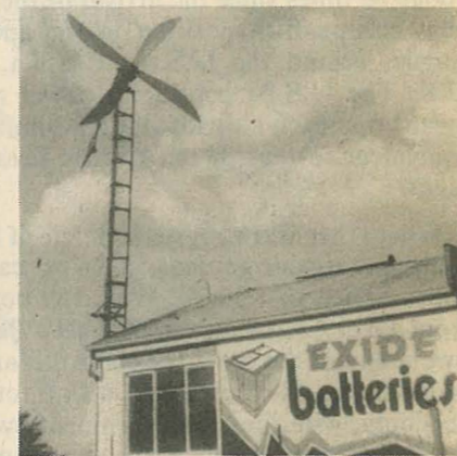
It's always good to see a wind generator actually working and being used, and here's one with a bright yellow prop that you can see in the back streets of Sunbury, atop Jeff Farmer's Sunbury Auto Electrical Service workshop. It's a 1 kW mill and Jeff uses it for charging auto batteries. The prop blades are hollow, made from tin sheet folded to form an aerofoil section.
