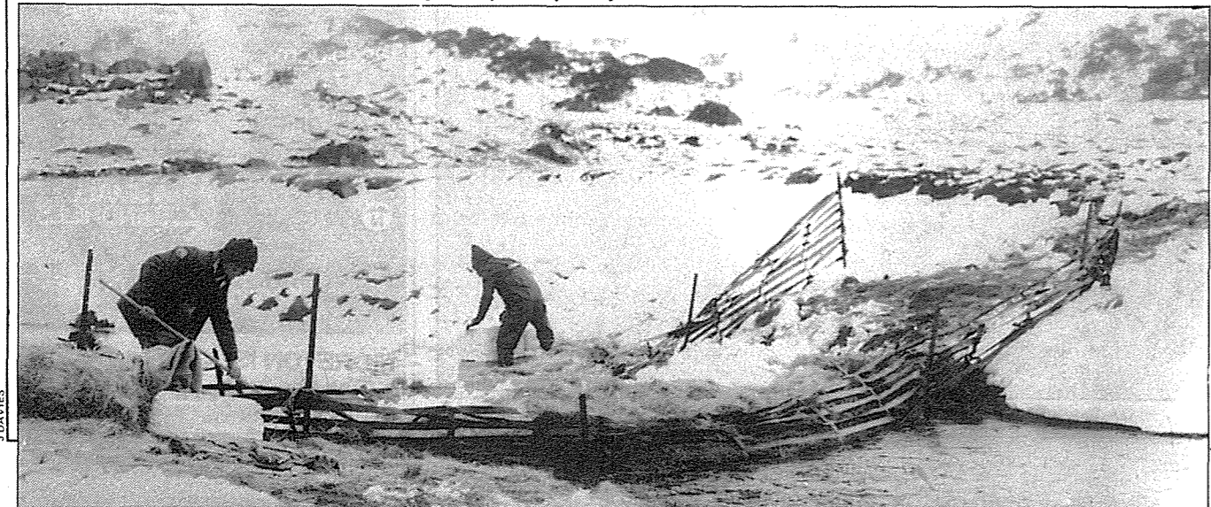
Dam building on Spencers Creek to stop the flow of oil pollution. June 1979
