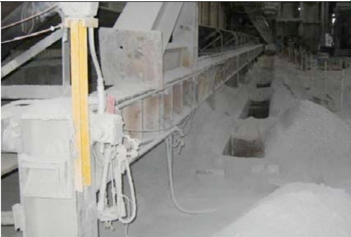
Photo No. 6: Fall Hazard from unguarded holes and dust accumulation
