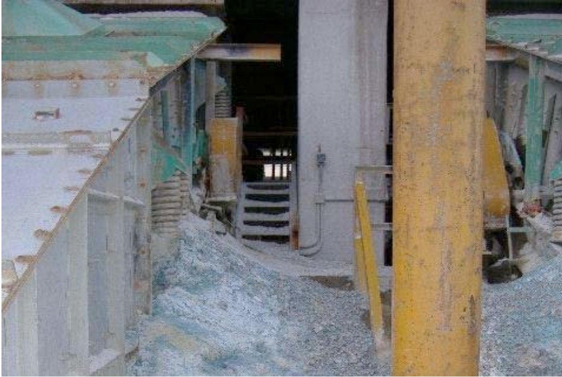
Photo No. 7: Working Surface – blocked exit passageway
