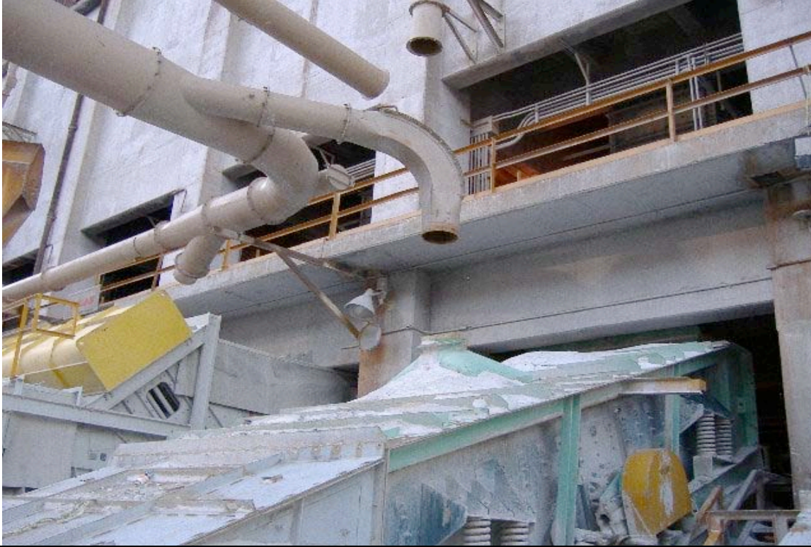
Photo No. 5: Disconnected exhaust ductwork to dust collection system
