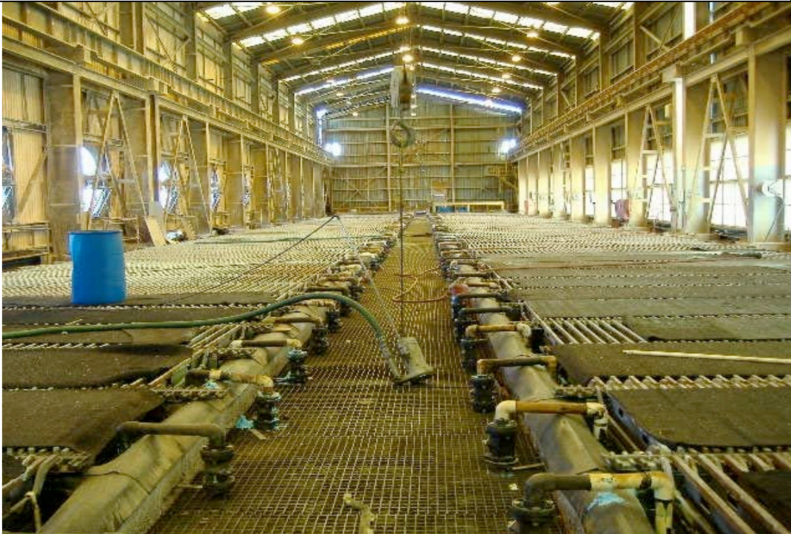
Photo No. 12: Acid mists and lead hazards in ESDE # 2 Building
