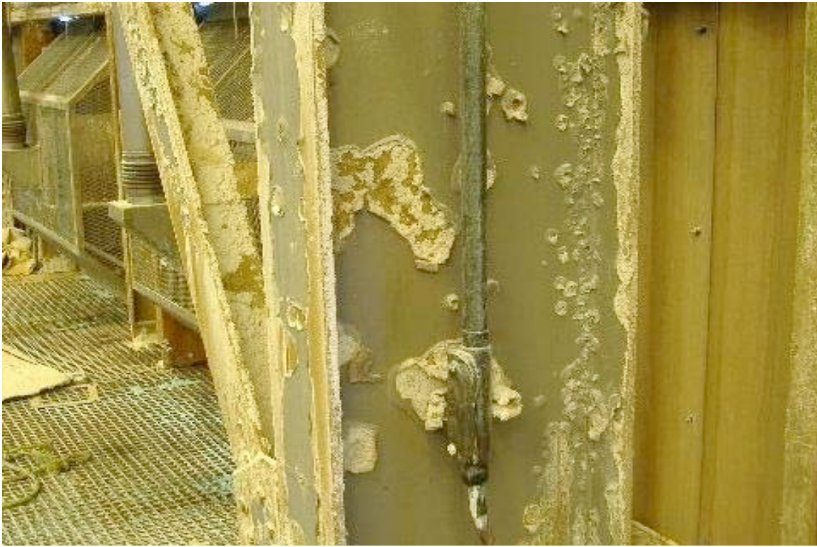
Photo No. 11: Chemical hazard: Corroded steel from acid mists in ESDE Building
