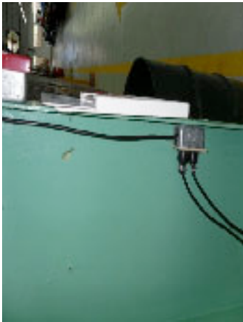
Located on east side of plant. Cord coming out from box has no protection from sharp edge of knockout.
