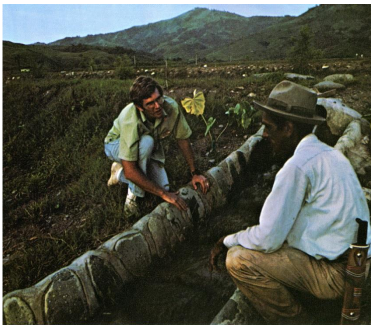
A Peace Corps Environmental Program volunteer and a local man discuss a new pipeline designed to provide drainage for an agricultural project in South America, 1973, photographer unknown, Smithsonian Institution Archives
